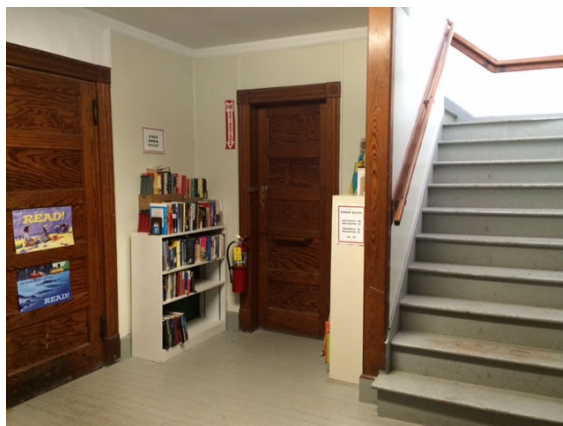
The anticipated installation of a vertical lift near the front staircase will allow access to the second floor of the Town Hall.
